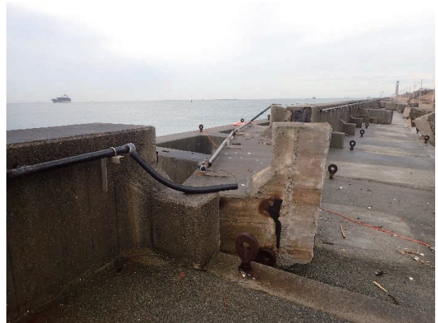
写真-5 夢洲護岸の破壊
